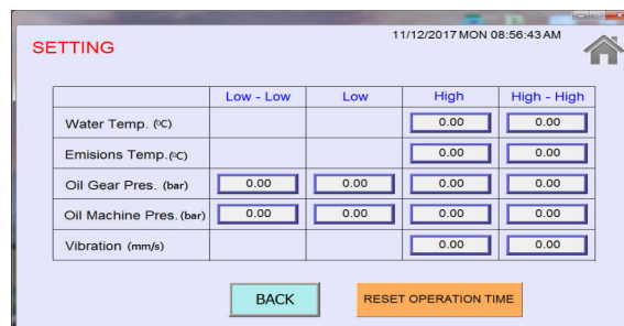
Fig. 4. Control program displaying monitoring parameters
