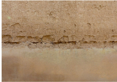
Figure 8. Surface erosion of adobe (Patrocinio, et al., 2020)
